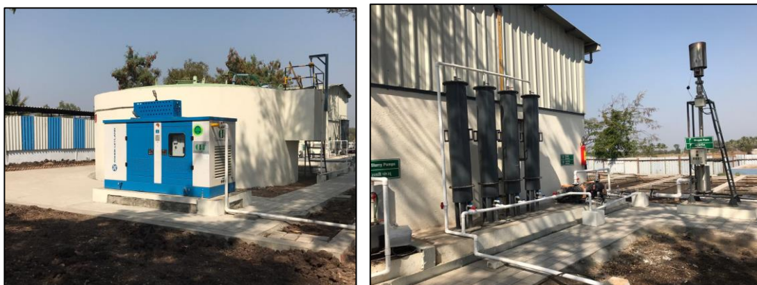
New Bio-gas facility at Tasty Bite that can take 4 tons per day of organic food waste
